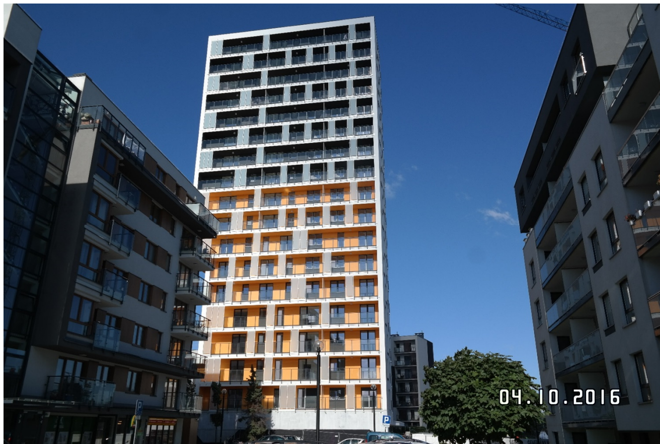
Building 6.4 (17th floors) on construction, Apartamenty Innova, Wrocław . On the right, building 3.2 and on the left, building 4 of Osiedle-Innova (October 2016).
