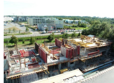
Ostoja-Wilanów, Warsaw, (stage 8, building B2). No. of units: 43 apartments plus 3 commercial units (4,968.4 sq. m) Breaking ground: March 2016. Progress to date: 30% (as at 30 September 2016). Delivery date: Q4 2017 On sale since: March 2016 (54% presold at 30 September 2016).
